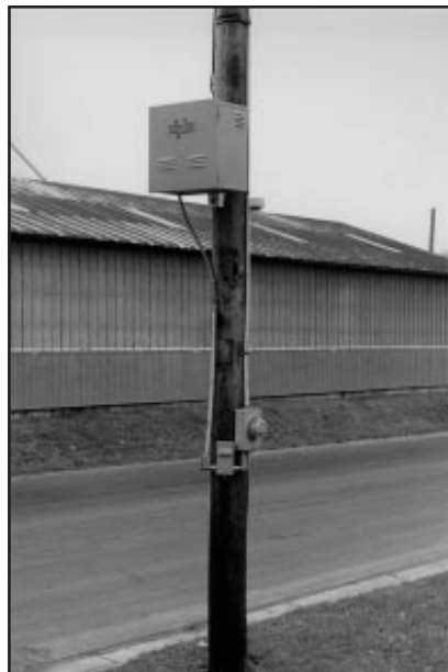
FIGURE 3. Typical pole-mounted power supply. Electric power, at 115 volts, is obtain from the power company's utility.
