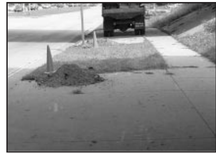
Figure 3. BEFORE: West Mineral Point Road facing east, before relocation of the WMSN and KMC fiber cables. The piles of dirt in the terrace at the left mark the location of the WMSN fiber. KMC's fiber is located behind the embankment to the right. WISDOT has ordered both companies to relocate their fiber cables to a new trench located near the sidewalk at the right.
