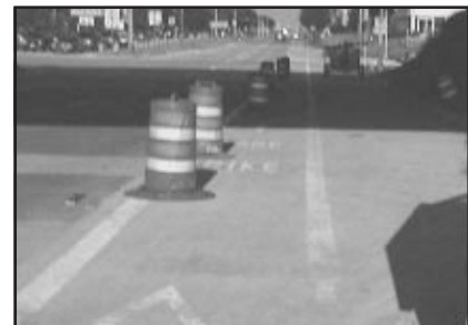
Figure 4. AFTER: West Mineral Point Road facing east, as of August 5, 2000. The old terrace is now a bicycle lane and the old sidewalk is now another traffic lane. Both fiber cables (WMSN and KMC) are now safely buried under the new traffic lane. The embankment to the right is still under construction; when the project is finished, the embankment will be replaced with a new sidewalk and retaining wall.
