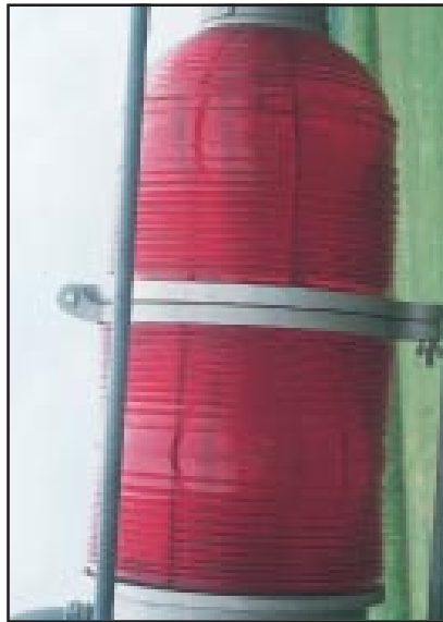
Figure 2. Flashing red beacon is hinged in the middle for relamping.
