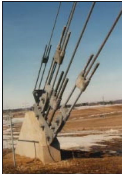
Figure 3. Large anchor connects guy wires to the ground.
