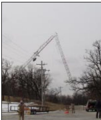
Figure 4. The tower bent in half and the top hit the ground.
