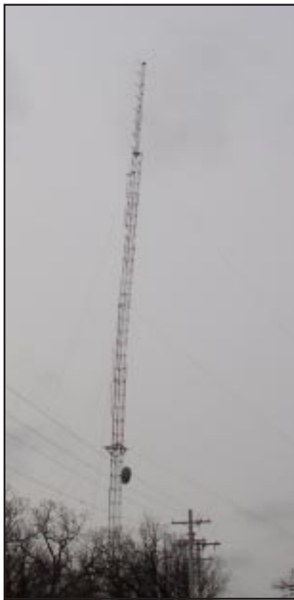
Figure 3. After the guy wire was cut, the tower began to lean toward the West.
