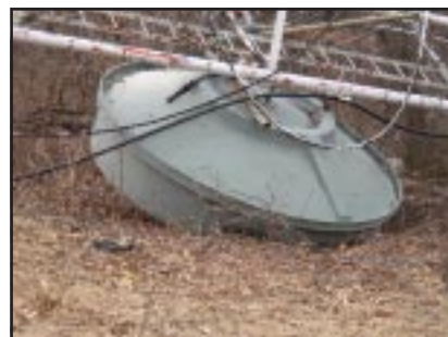
Figure 10. Microwave dish crushing inward.
