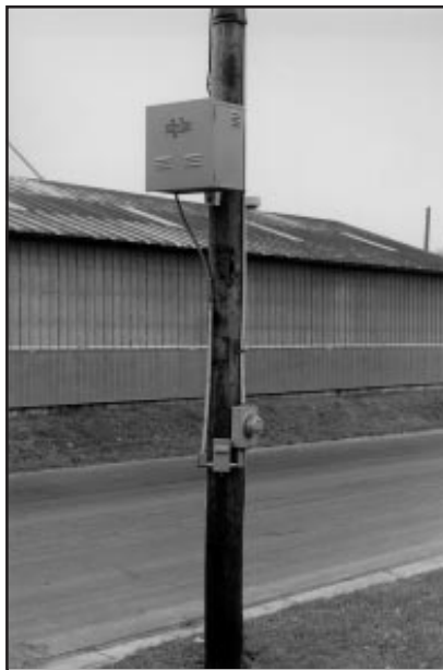
FIGURE 3. Typical pole-mounted power supply. Electric power, at 115 volts, is obtain from the power company's utility.
