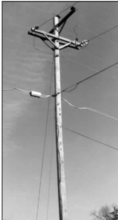
Figure 3. A CATV trunk amplifier on a joint utility pole. The amplifier is the strand-mounted device just to the left of the pole. This particular pole is located on a side street so that a bucket truck parked near the pole doesn't block traffic.
