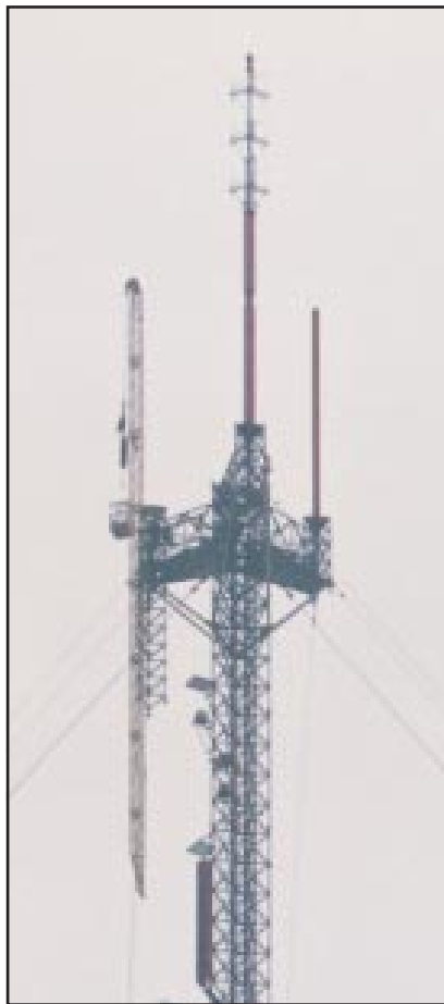
Figure 2. Gin pole mounted on left side of Candelabra is used to raise antennas into place.
