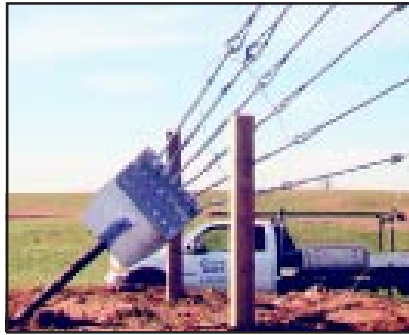
Figure 4. Guy anchor for WSUM tower. (Figure 4) was manufactured by PiRod, Inc. Designed to withstand a 90-mph wind load, the tower meets the standards of the latest revision of the ANSITIA/EIARS-222-F code. The tower has the capacity to hold many cellular and PCS antennas, in addition to WSUM's antenna.
