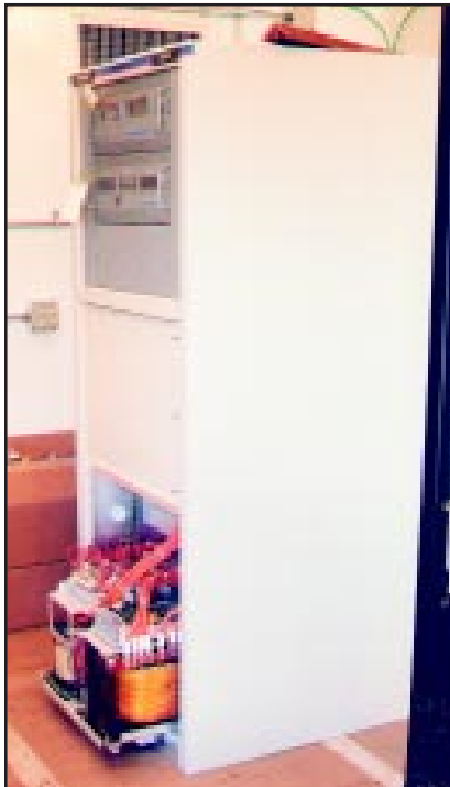
Figure 3. WSUM transmitter. From top to bottom: metering, exciter, IPA module, and power supply.
