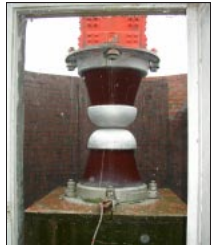
Figure 2. The porcelain insulators at the base, which support the entire weight of the structure, are predicted by one expert to support in excess of 300 tons. A very large spark gap (not shown) is behind the insulators.
